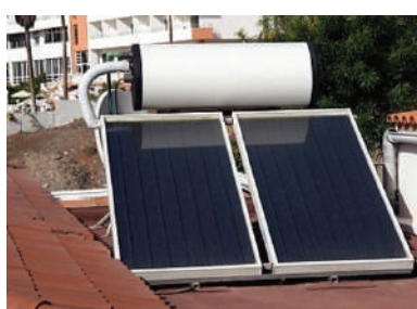
Fig. 12.3 Solar flat plate collector
